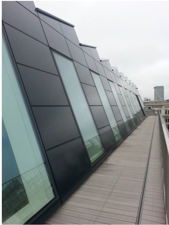
Solar panels integrated into a Mansard Roof
